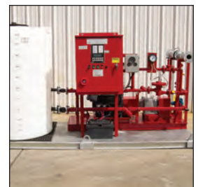
Diesel Pump Skids
